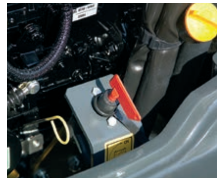
The battery main switch is standard
